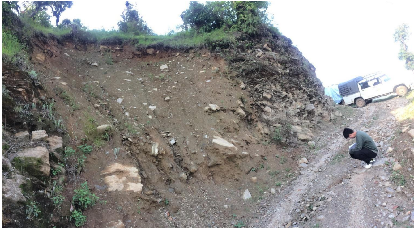
Figure 8: Picture showing landslide due to road cut
