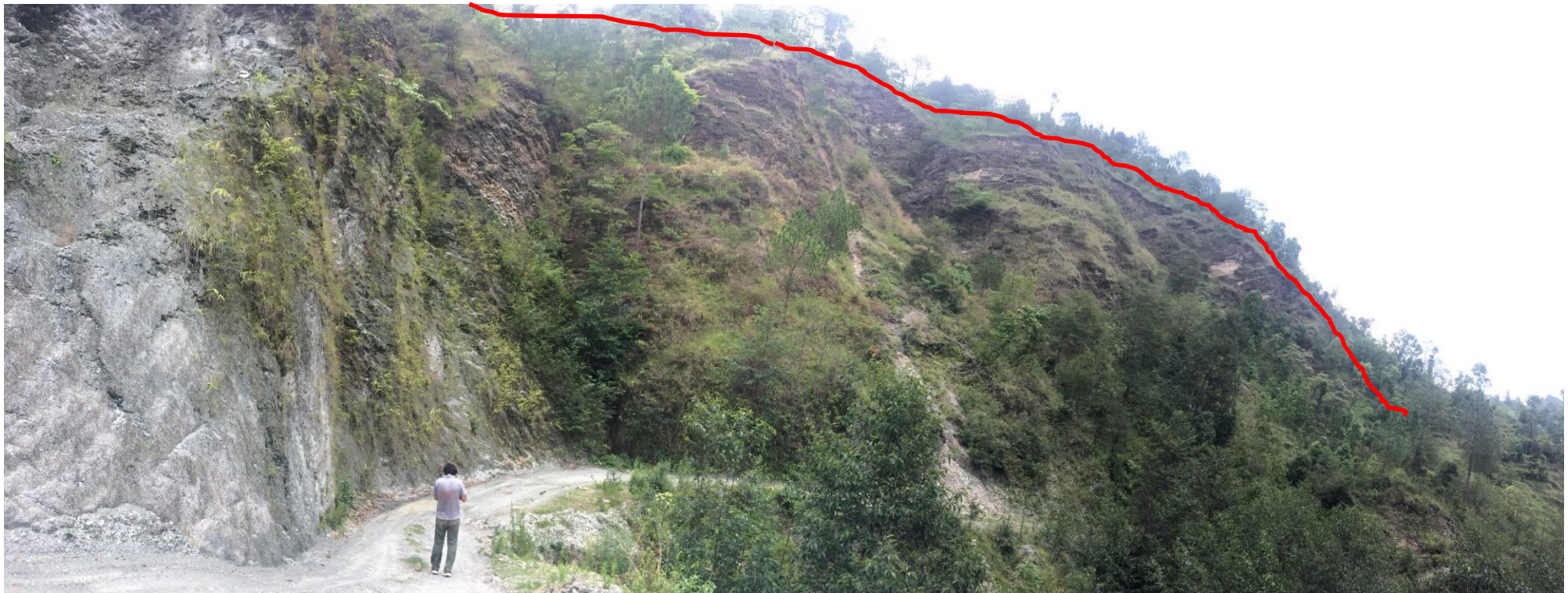
Figure 12: Picture showing old landslide, existing road, and reactivated debris flow
