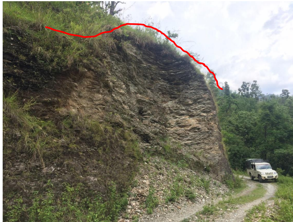
Figure 13: Picture showing road cut, and highly weathered rock leading to debris flow
