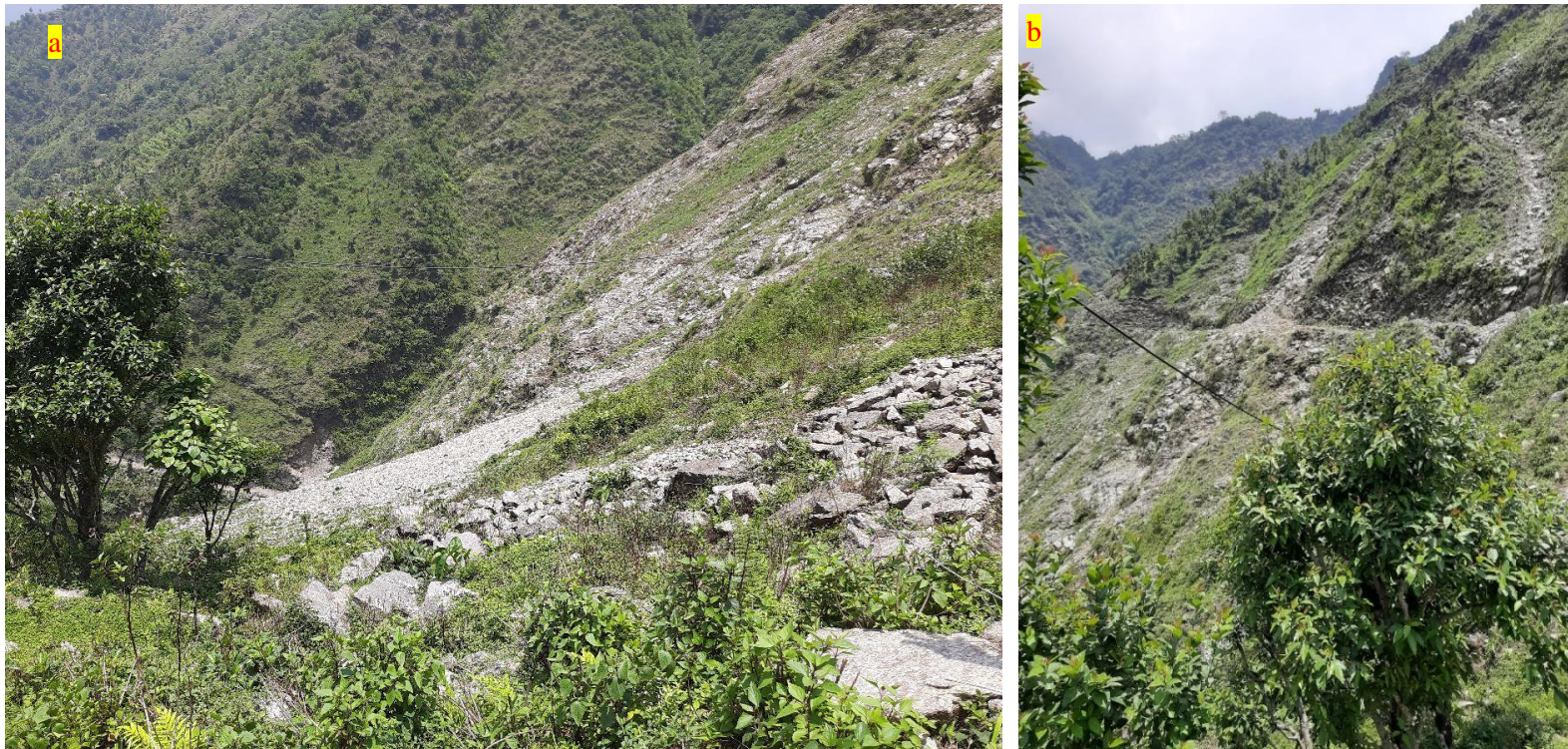
Figure 7: Picture showing debris flow from the landslides(a) downslope (b) along the road cut
