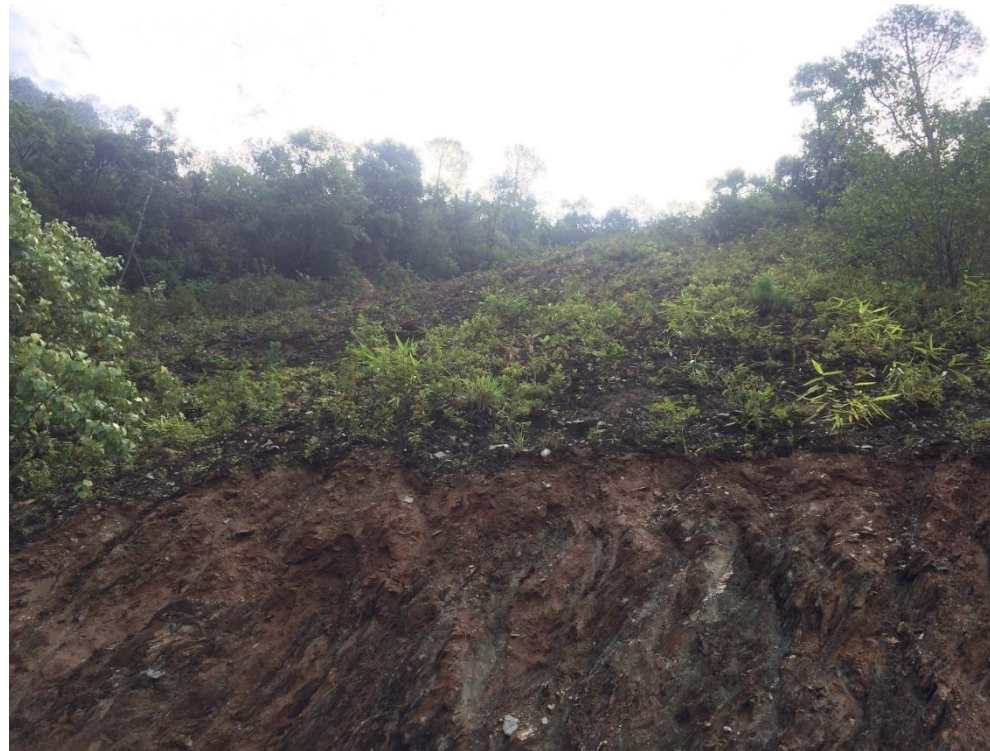
Figure 10: Picture showing shallow landslide at Khimli
