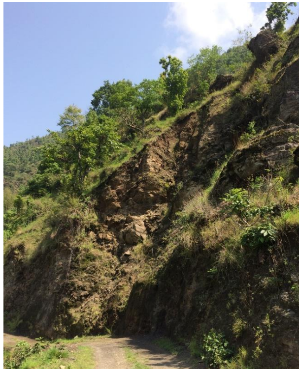
Figure 6: Picture showing Landslide on upslope of road
