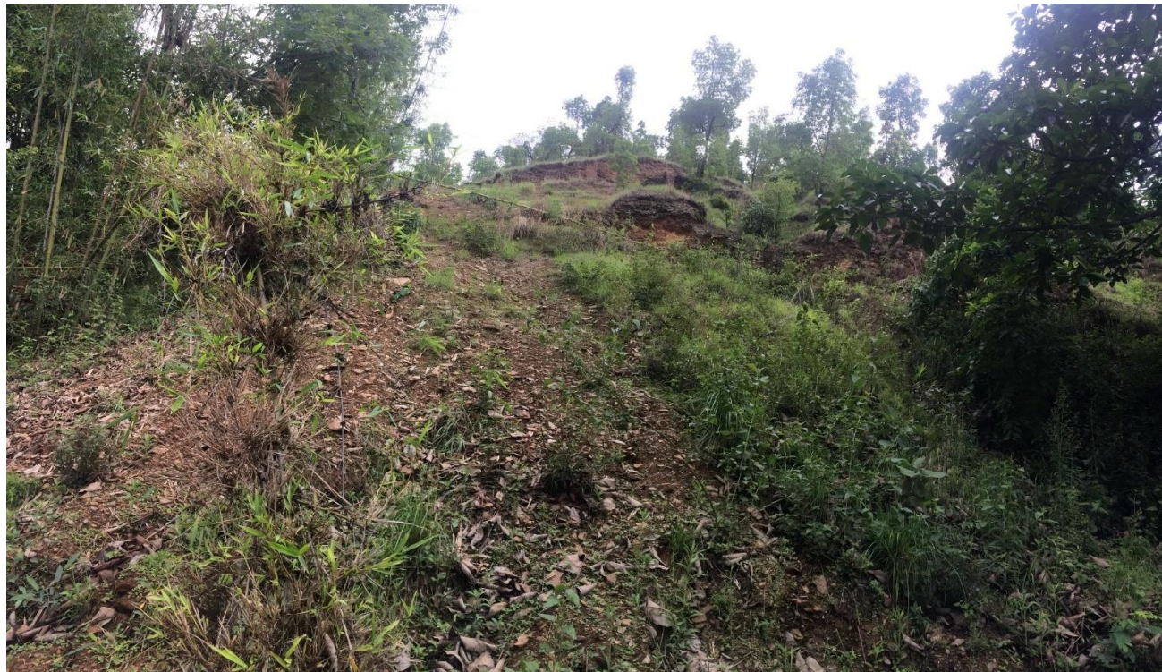
Figure 16: Picture showing shallow landslide with vegetative growth
