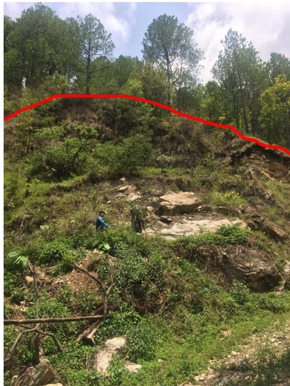
Figure 24: Picture showing landslide with mud fall
